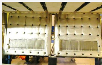
heat shields to reduce heat loss
